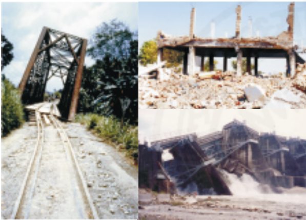
Fig 2.1.4 shows the adverse effects of an earthquake
