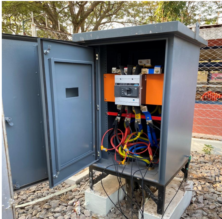
Fig: Incoming Supply Bus-Bar installed at campus
