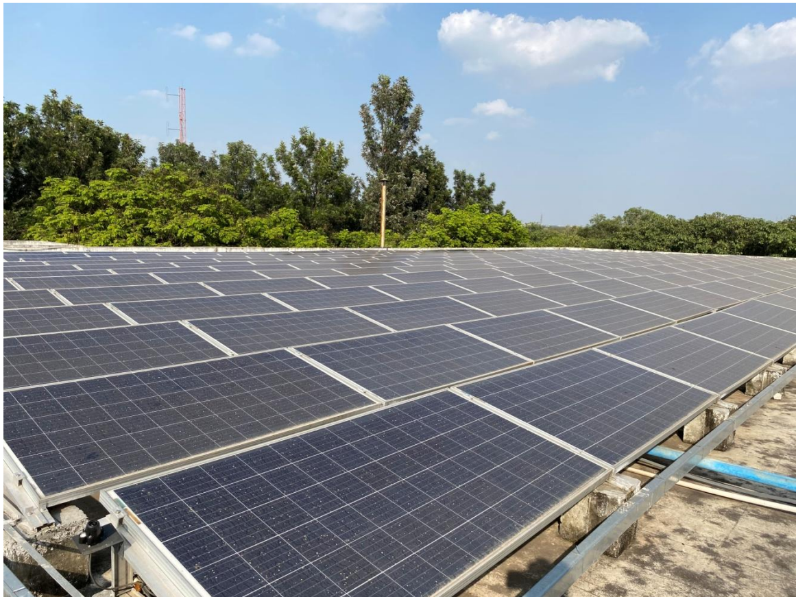
Fig Shows Solar Panels installed at campus.
