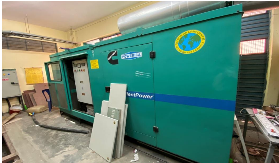
Fig: Name Plate Details of Cummins Diesel Generator installed at campus
