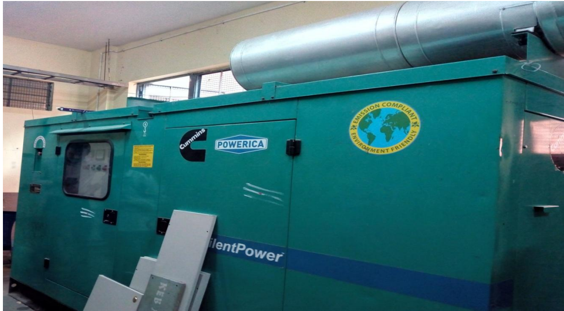
Fig. 100 kVA Cummins Diesel Generator
