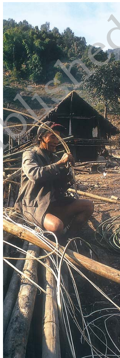
Fig. 5 – A log house being built in a village of the Nishi tribals of the Northeast.
