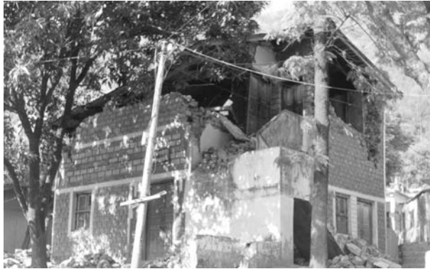
Figure 7.1 : A Damaged Building Due to an Earthquake
