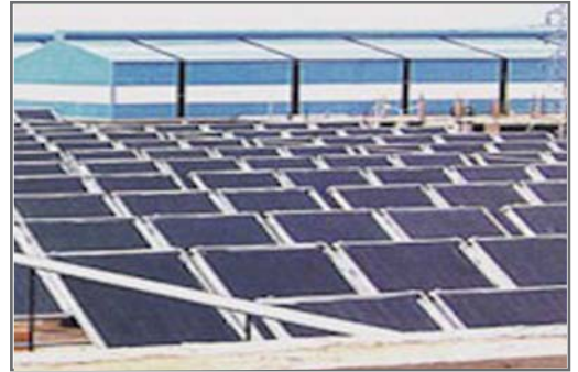
Fig 3.17: Solar Panels to trap solar energy
